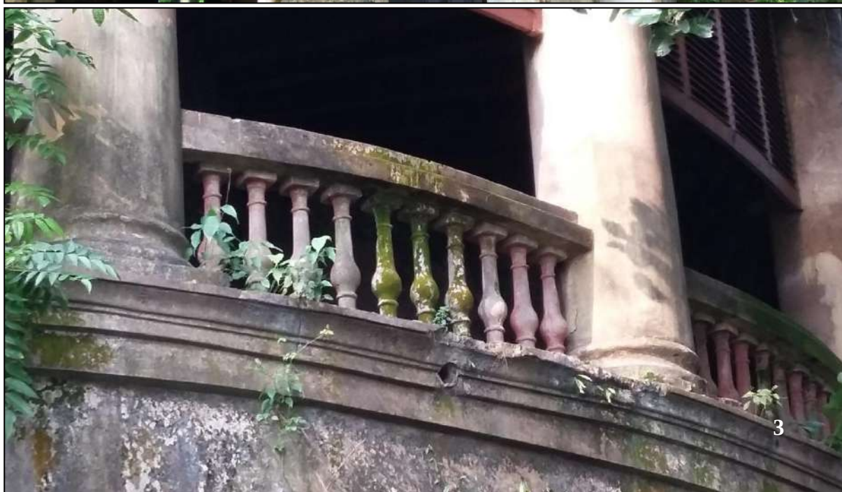
Photo 2 & 3 Algal patches on Roxburgh Building
