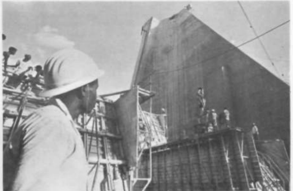
Constructing the Rosettes dam across the Blue Nile with the help of World Bank financing
