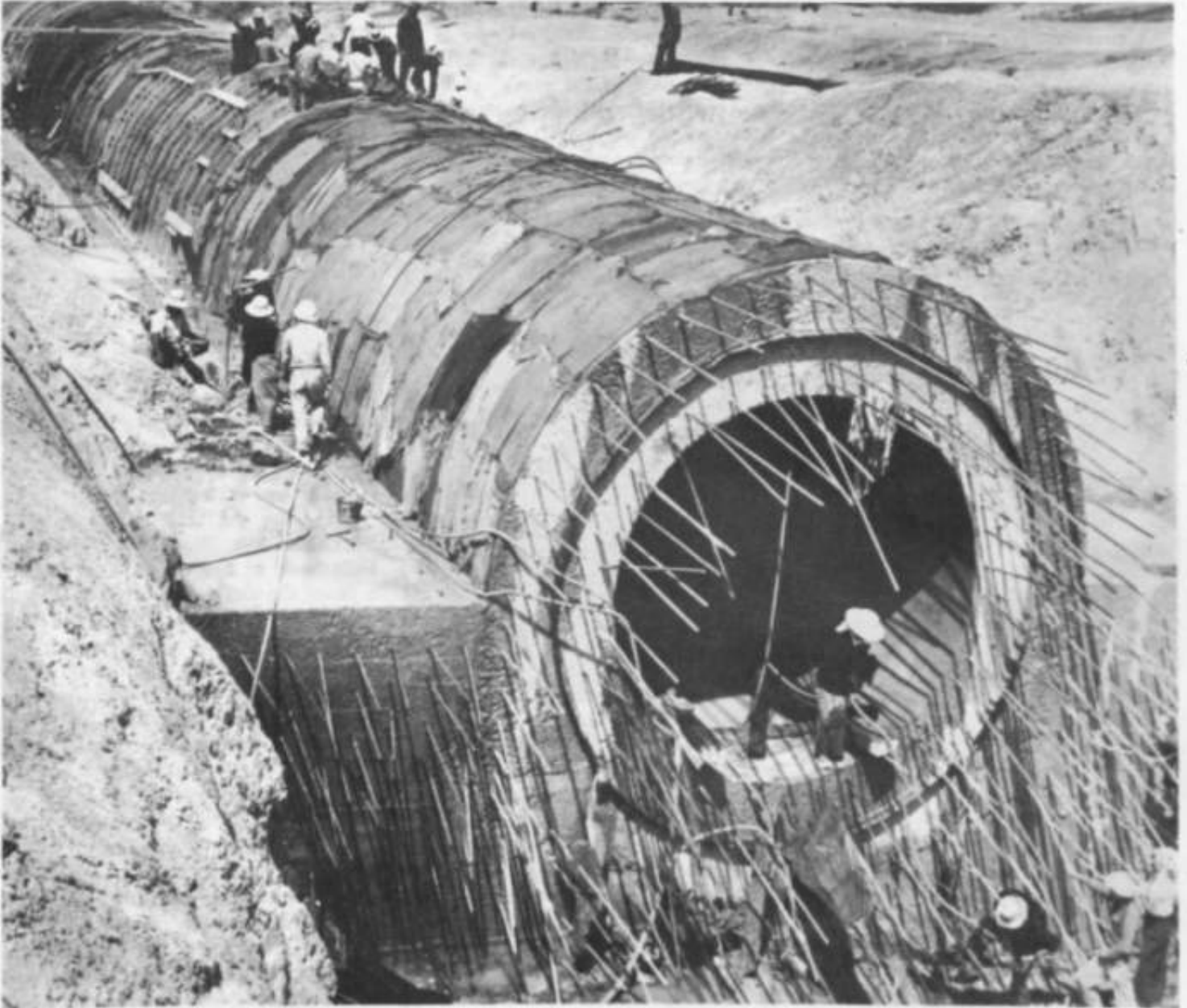
Waier for new areas of Irrigation i/t Thailand. Here, a large upsuetm conduit undei construction some years ago as part of the Marty Kiactiar* dam complex on tn$ Petchbun River tinancett by a $3.4 million loan from the World Bank.
